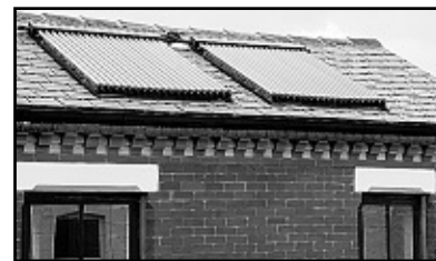
WATER POWER: The solar thermal evacuated tubes panels on the roof
